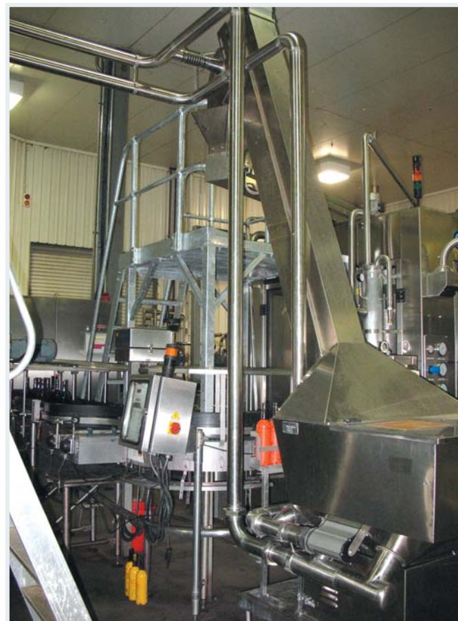
Hopper, elevator and air knife, and exhaust air piping
